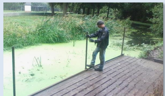
Mark making sure the scaffold poles on the landing stage are secure
